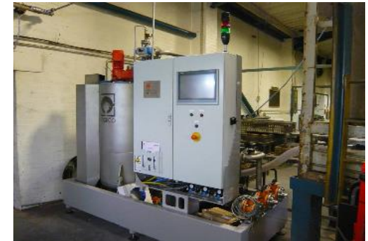
Intelligent Coating Unit
