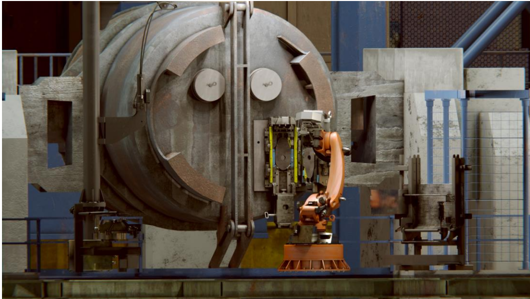
New Flow Control robotics solution for ladle make-up area
